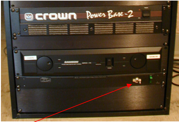
Equipment Cabinet Power Switch (Toggle) Figure 3
